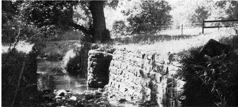
General view of the right-hand wall of structure in the Castle Beck, showing circular protrusion, with the slots in the wall at the farther end (Courtesy D. G. Tucker)
